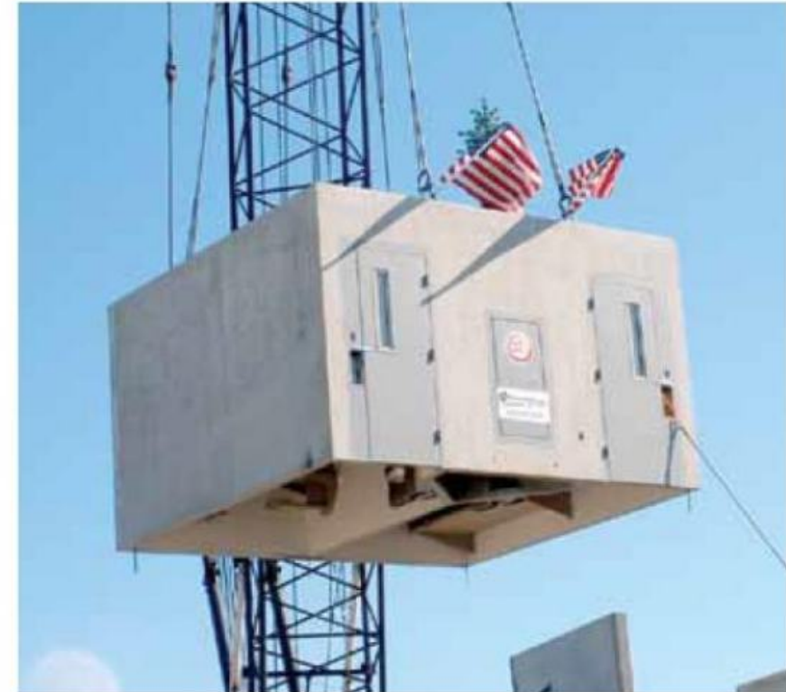
Fig. 1.2.16 A precast concrete double-cell module is lifted into place, complete with furnishings installed.
